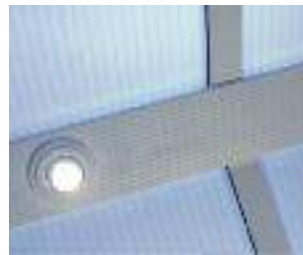
Lighting - integrated downlighting in the roof ridge space and pelmet surround.
